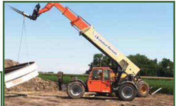
Brother Richard French operates a JLG Forklift while setting forms for Mortenson at the Pocahontas Prairie Windfarm
